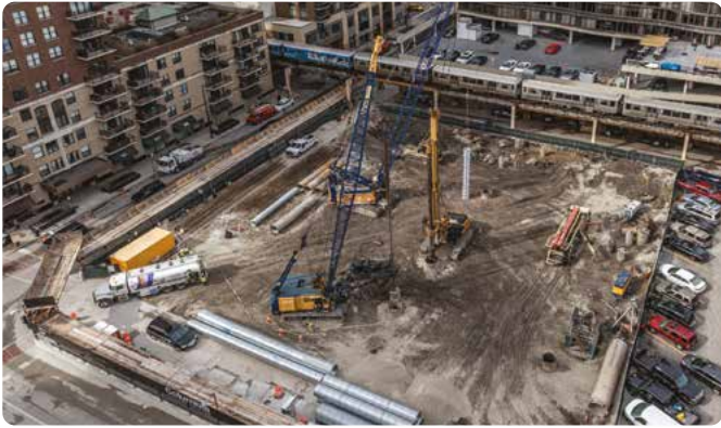
Columbia College's new student center abuts an elevated train track, presenting challenges for the construction team. Photo © Ballogg Photography.
