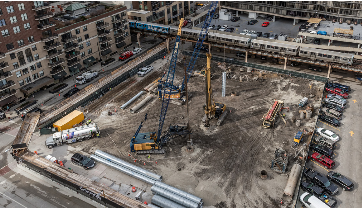
Columbia College's new student center abuts an elevated train track, presenting challenges for the construction team. Photo © Ballogg Photography.
