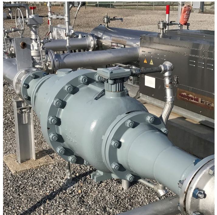
Field installation of a Brodie 8 inch Birotor Plus meter
