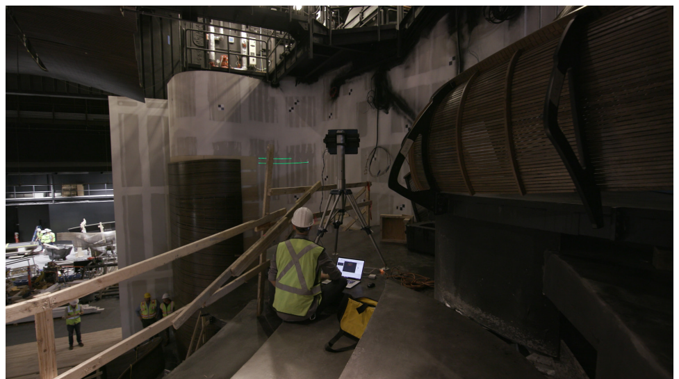
The CWKA team used the Tracer in combination with FARO BuildIT Construction software to project panel templates onto theatre walls.
