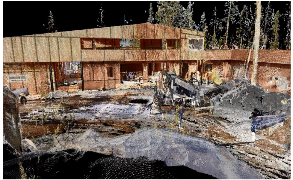
Scan data of the project saved time, reduced risk and provided confidence across the team.
