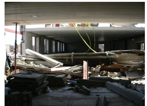
Figure 5. Under construction seven-story building with a 100-foot by 250-foot footprint that collapsed when it had been built up to five stories.
