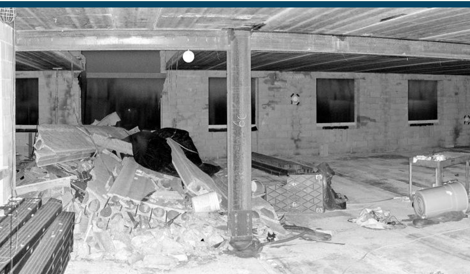
Figure 1. Point cloud data of an under construction seven-story building with a 100-foot by 250-foot footprint that collapsed when it had been built up to five stories.
