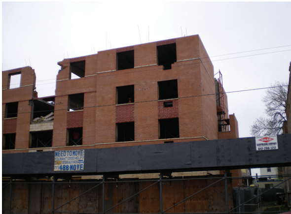
Figure 6. Photo of the collapsed building under construction.
